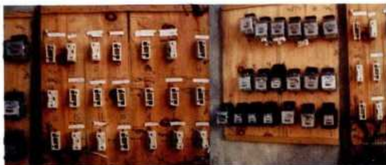
Inside view of power house in which they fixed meters and fuses.
