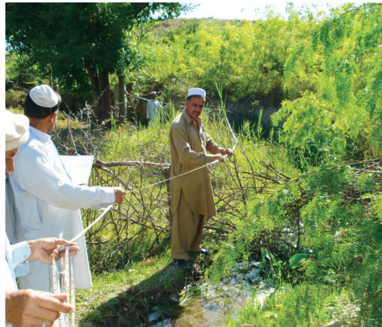
Technical Support provided to MCO Sro Gharugo 1 during survey for lining of water course in Lower Kurram (Kurram Agency, August 2009)
